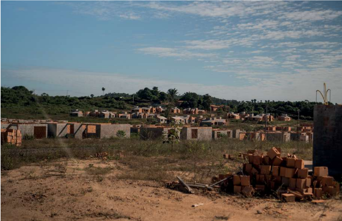
Image of houses for the resettlement for the community of Piquiá de Baixo, Açailândia/MA, June 2021.
